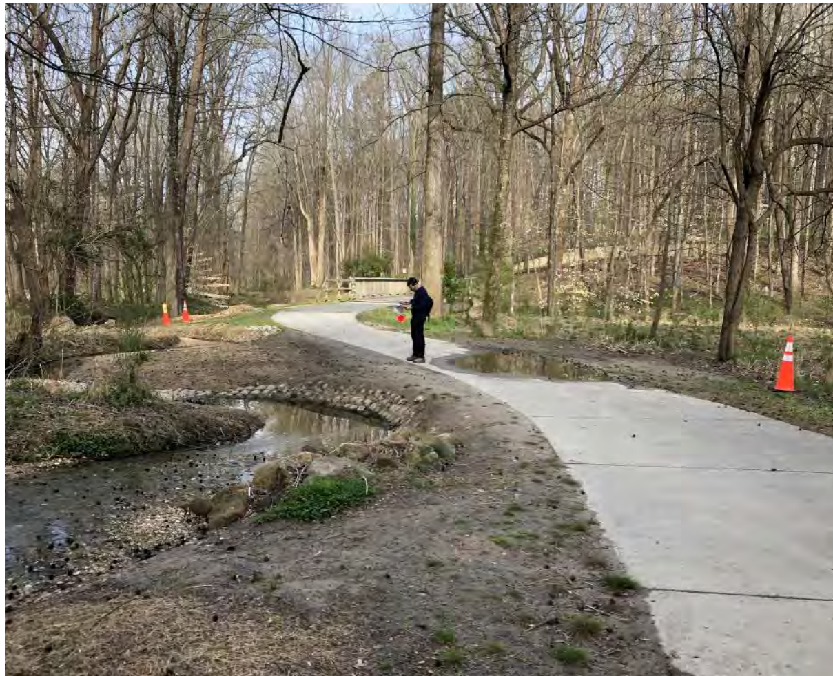
Unnamed tributary eroding banks and overtopping greenway to reach natural floodplain; Photo: Andropogon
