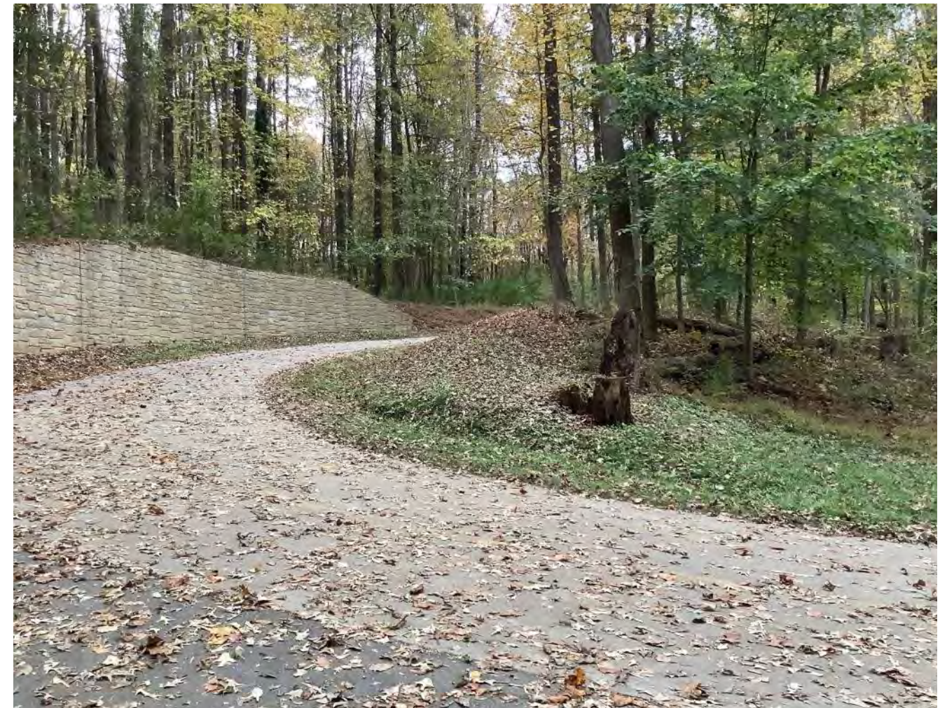
Greenway slope and curve not in compliance with AASHTO standards; Photo: Andropogon
