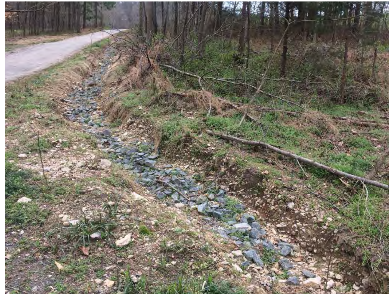
Erosion caused by concentrated runoff from Lower Meadow; Photo: Andropogon
