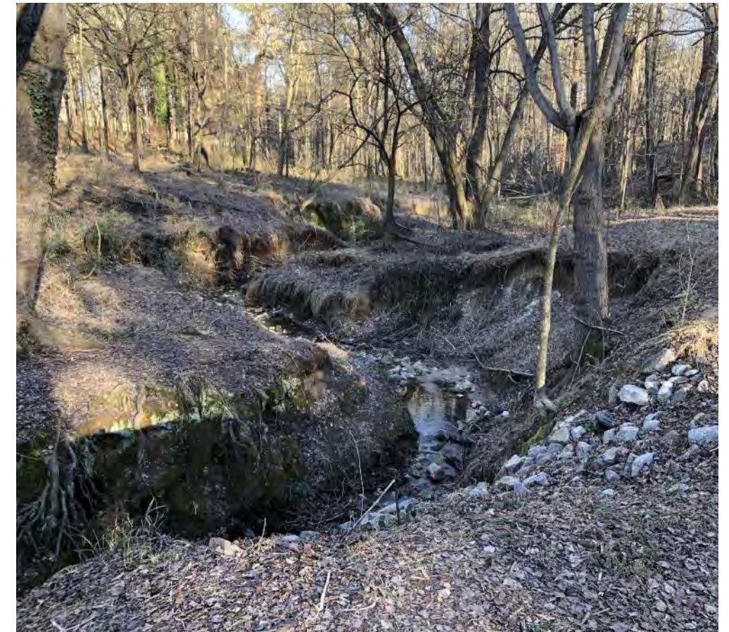
Erosion just downstream from Blue Loop crossing (February)
