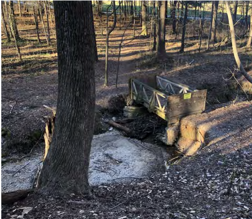
Blown-out bridge at forest path crossing (February)
