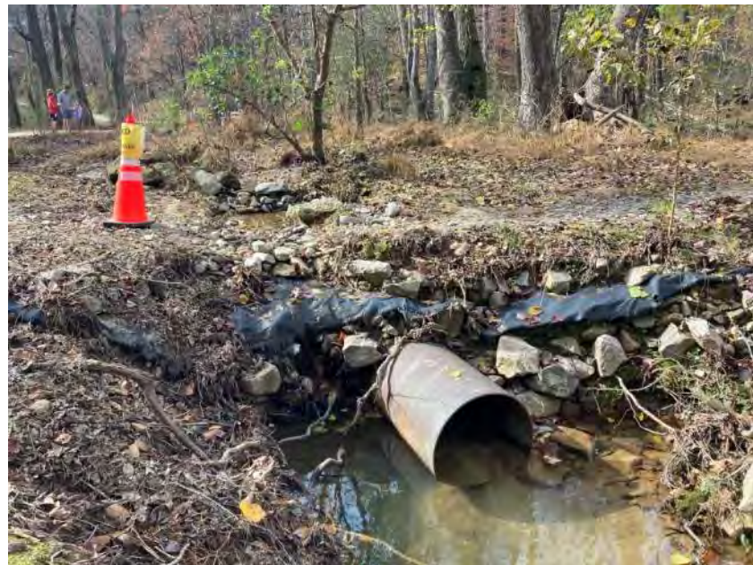
Photo 4. Failed 24" DIP culvert at Sta. ~1+30 (WKD 2020-11-29)
