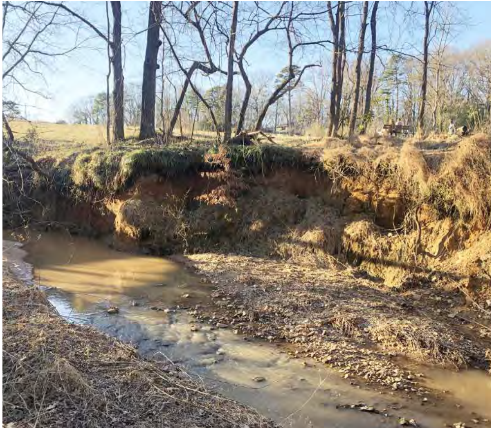
Erosion below seating area and trail in Lower Meadow (February)
