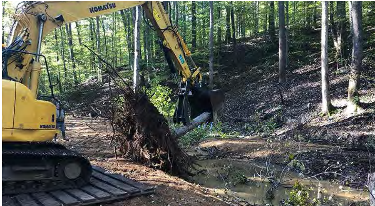
Construction: placement of a root wad to raise the stream invert level
