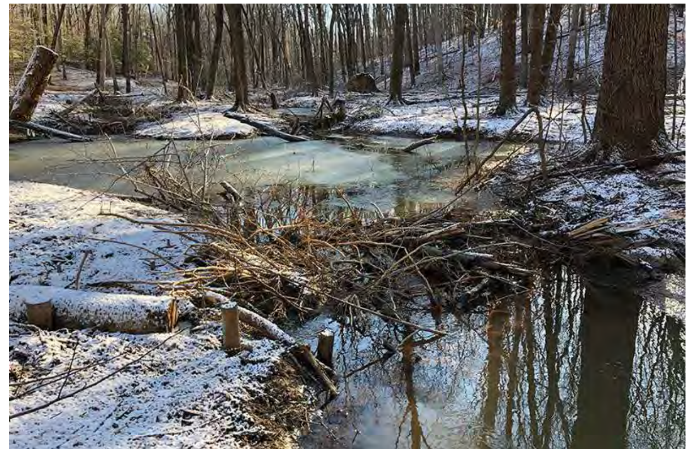
Postrestoration: woody debris and log jams constructed from wood harvested on site
