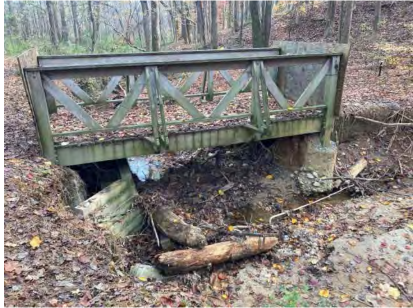
Photo 3. Abandoned footbridge at Sta. 11+75 (WKD 2020-11-29)
